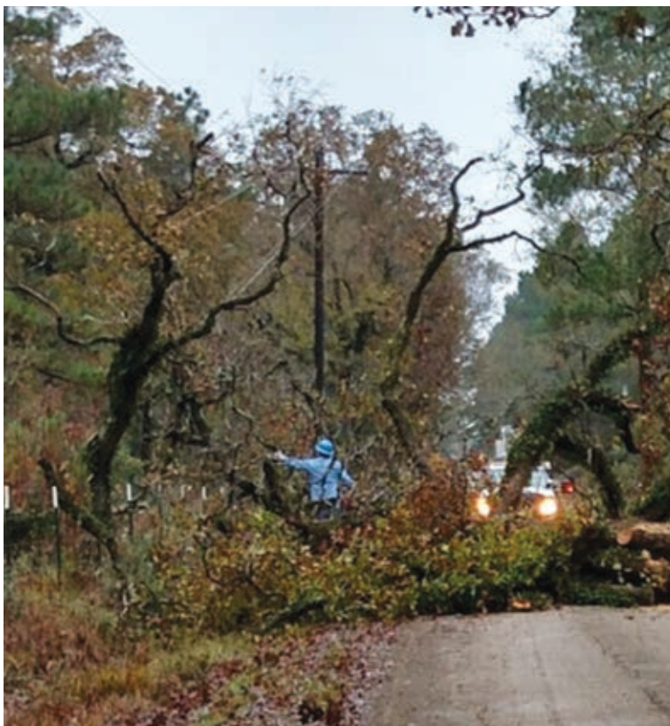
Houston County EC member Kelly English captured this photo of an HCEC lineman working to clear downed trees following a storm.
